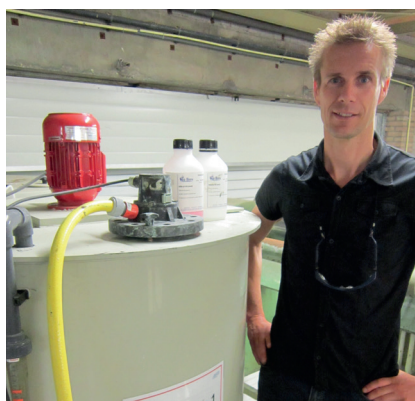
Luc Heldens in front of the 2 cyanide oxidation tanks
