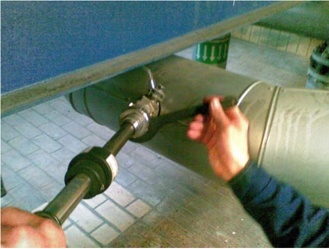
Oxygen sensor Oymax COS22D is brought into the process with the Cleanfit CPA450 assembly.
