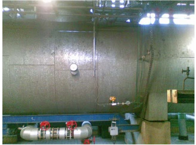
Thermal degasification at EC Lublin Wrotkow.
