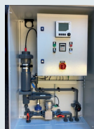
Wash Water Monitoring System (pH, TU and PAH)
