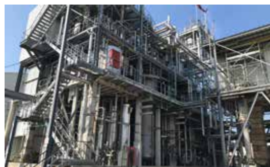
Scrubber at the Proviron plant in Oostende, Belgium
